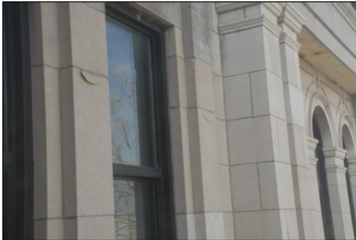
Stone ready to fall off exterior
