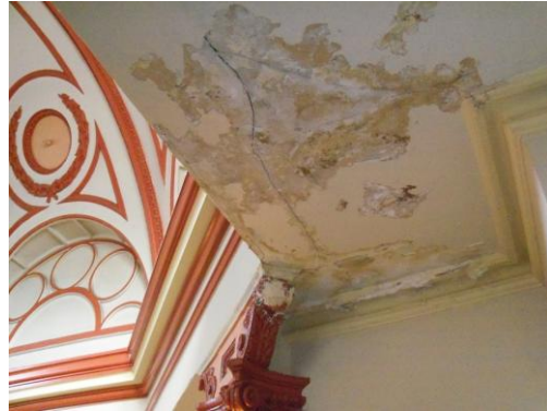
Water damage on the 4 th floor
