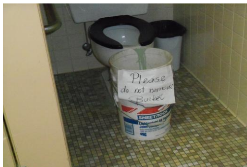
4 th floor restroom bucket for roof leak
