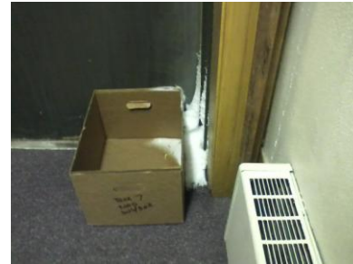
Snow blowing under fire escape door
